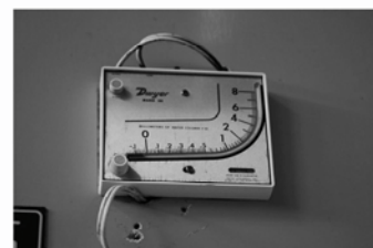
緩衝室之壓力計控管
